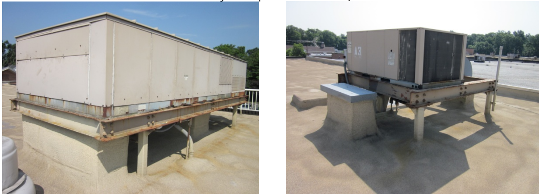
Chatham High School Rooftop Units
