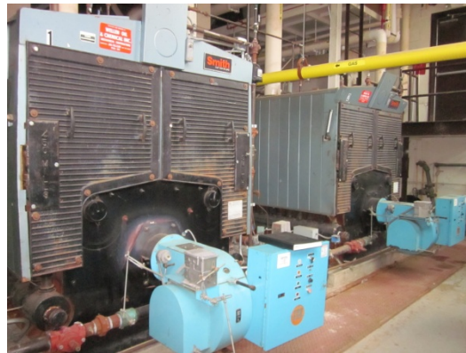
Chatham M.S. –Boiler Burners
