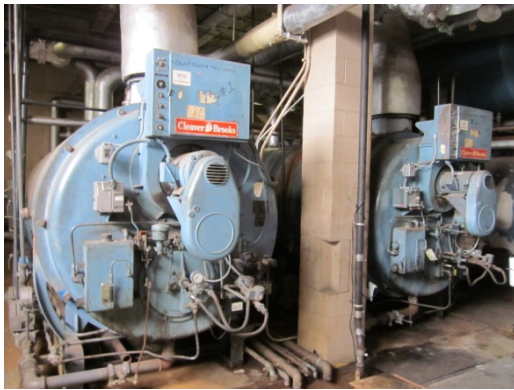
Chatham High School – Boiler Plant
