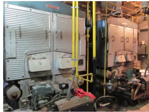
Southern Boulevard School – Boiler Plant
