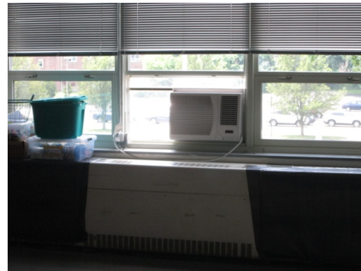
Window AC Unit in Classroom with Unit Ventilator Chatham Middle School
