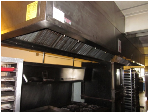
Kitchen Hood. Chatham High School
