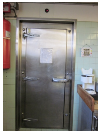
Walk-In Refrigerator. Chatham MS
