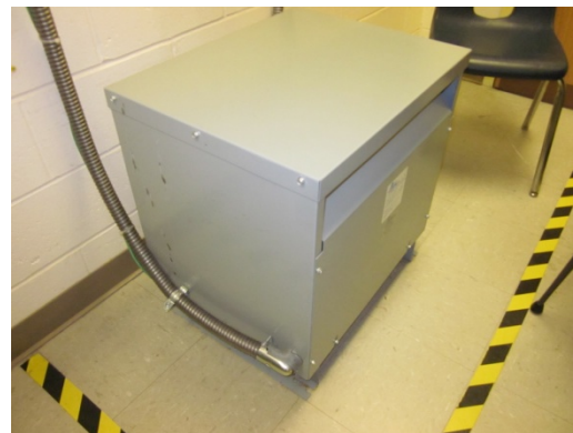
Transformer at Washington Avenue School
