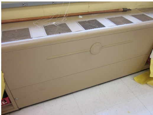
Washington Ave School – Steam Unit Vent
