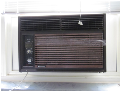
Older Window AC Unit in Classroom Chatham Middle School
