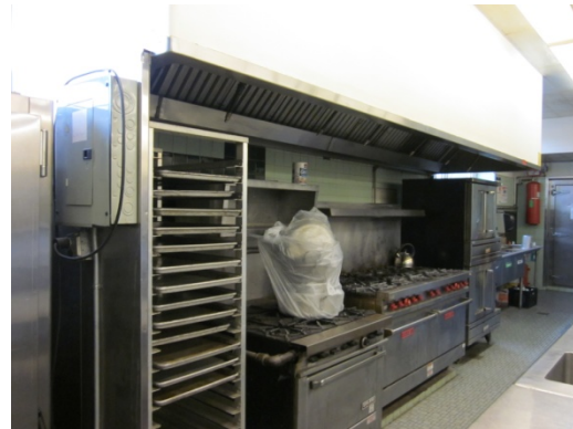
Kitchen Hood. Chatham Middle School
