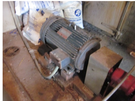
Chatham High School Hot Water Pump
