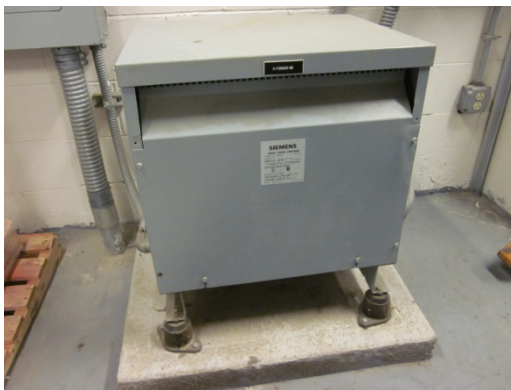
Transformer at Chatham High School
