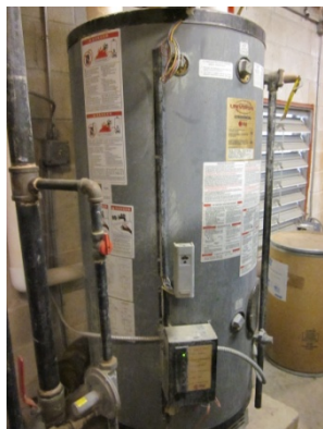
Southern Boulevard School DHW Heater
