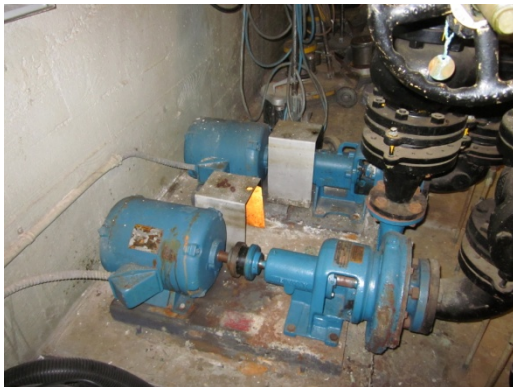
Southern Boulevard School Hot Water Pumps
