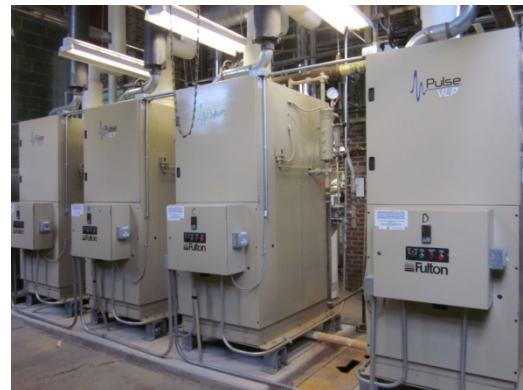
Milton Ave School – Steam Boilers
